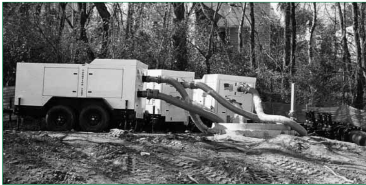
A 6 in. compressor-assisted open trash/sewage pump with a sound attenuated canopy on a site trailer.
